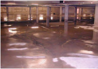
Fig. 1. Leaking floor in an underground parking house due to ignoring the effect of imposed deformation
