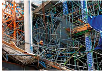
Fig. 2. Collapse of a shopping centre under construction due to an unstable scaffolding system
