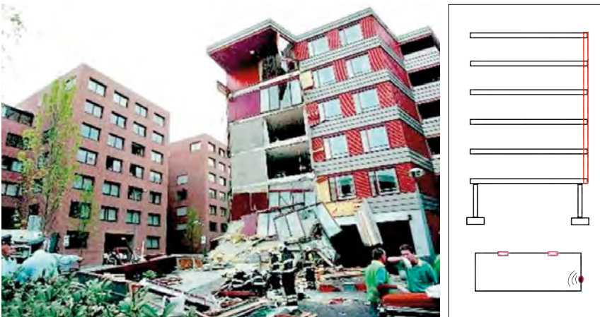
Fig. 4. Progressive collapse of a series of balconies in a high rise building, Maastricht 2003
