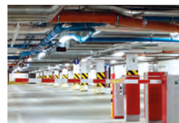
Fot. arch. Green Center
